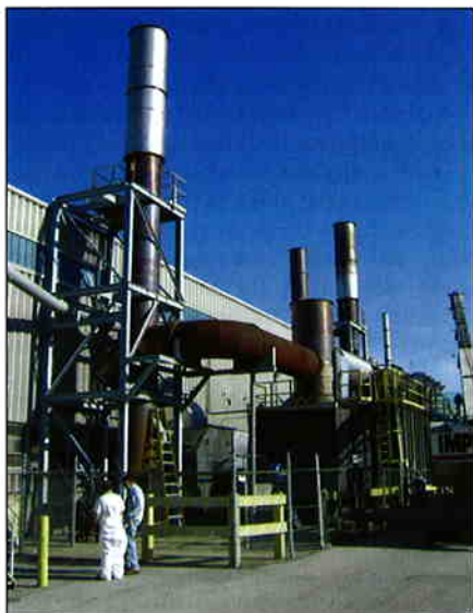
Silgan's aging thermal recuperative oxidizer was replaced by Anguil Environmental Systems
