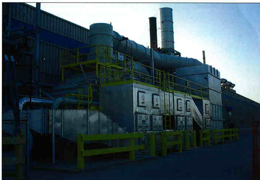
Silgan's chose its new regenerative thermal oxidizer based on the capital cost advantage and operating cost savings
